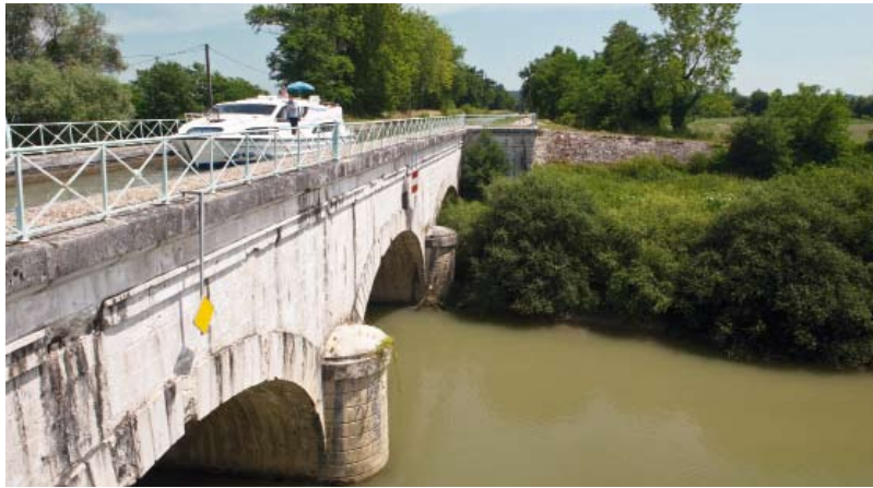
The Magnifique on the Pont-canal sur la Baise over the River Baise. Access to the River Baise is possible at Buzet
